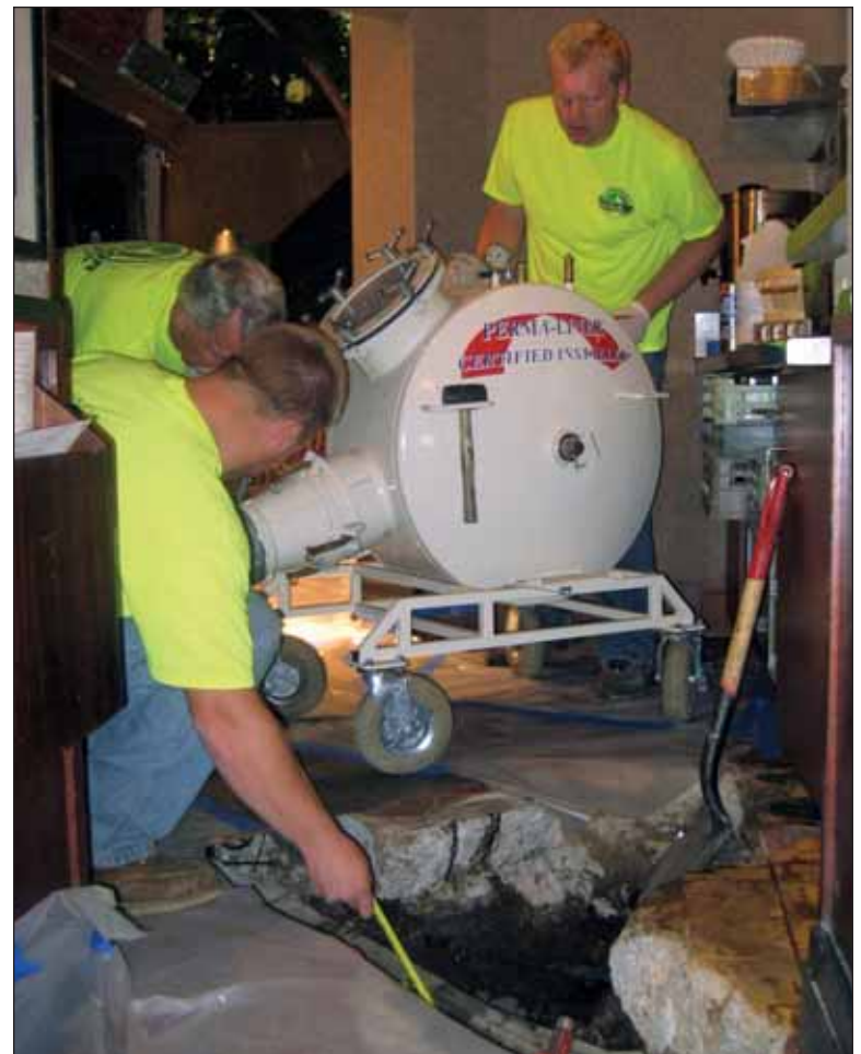
Troy Ouverson (standing) and Doug Ouverson position the air inversion tank as Scott Veal measures the distance from the tank to the pipe about to be lined. (Photos from Troy Ouverson)
